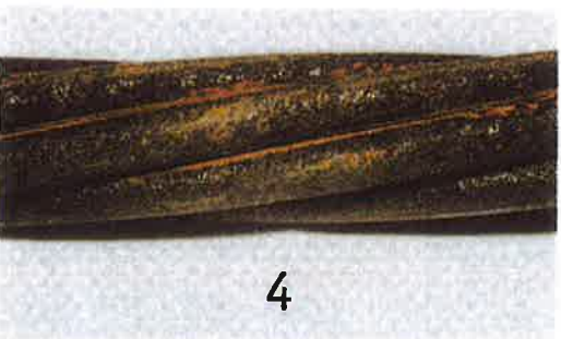
Photo 4. Strand surface before cleaning
